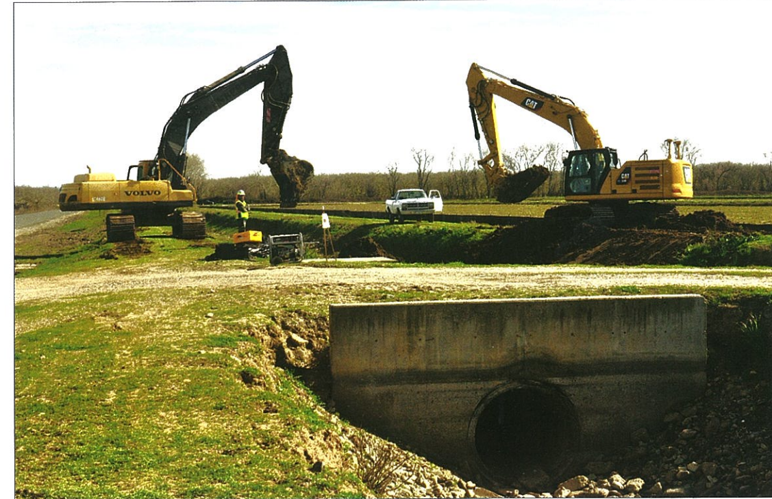
Two backhoes appear ready to dance with each other as they reshape a canal by giving the banks a gentler slope. One of the requirements during construction like this is for a biologist to remain onsite and be available whenever work is performed. The reason for the onsite presence is to ensure that if a displaced giant garter snake is uncovered through the work of the backhoes then the biologist will be available to relocate the snake to a safe area.
